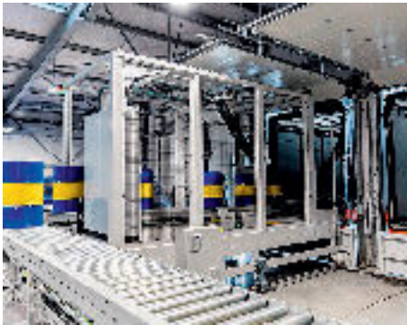
Empty barrels are fed fully automatically to the filling system with the aid of conveyor technology
